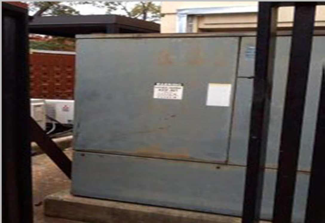
View of the pad-mounted electrical transformer at the subject property
