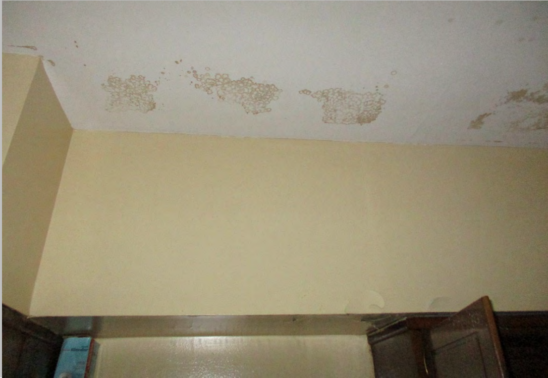
View of typical moisture intrusion in Unit 4E
