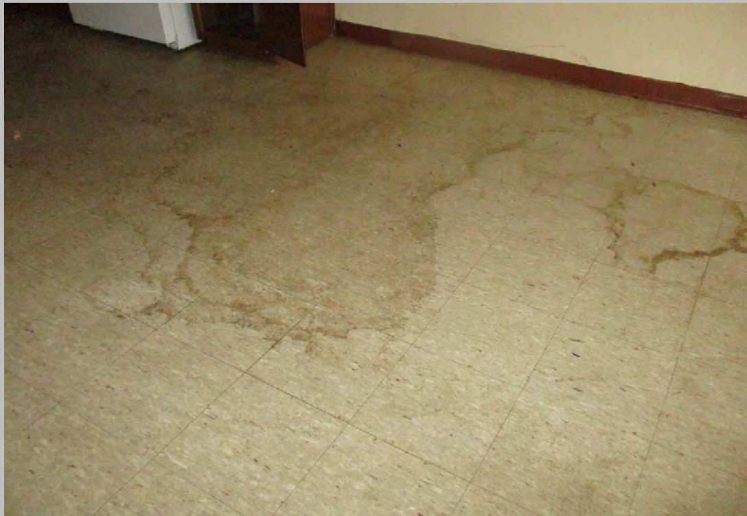
View of typical moisture intrusion in Unit 11F
