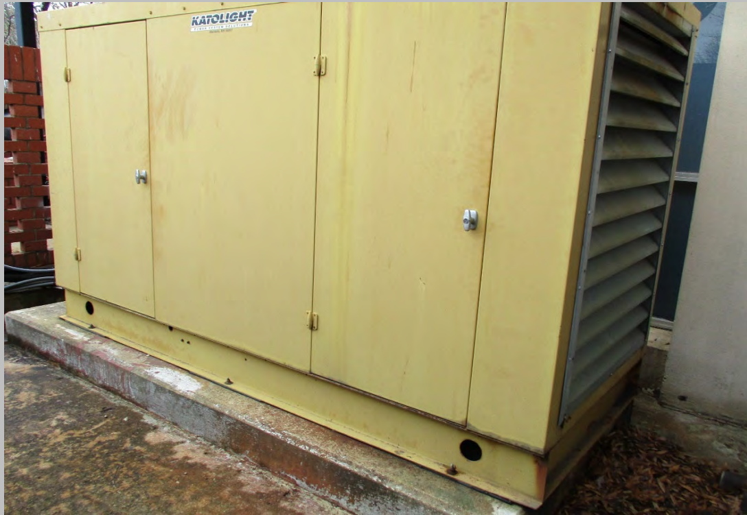
View of the natural gas generator at the subject property
