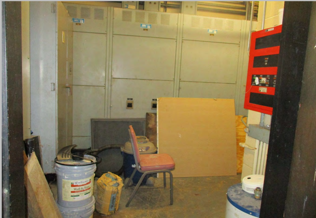
View of the electrical equipment area
