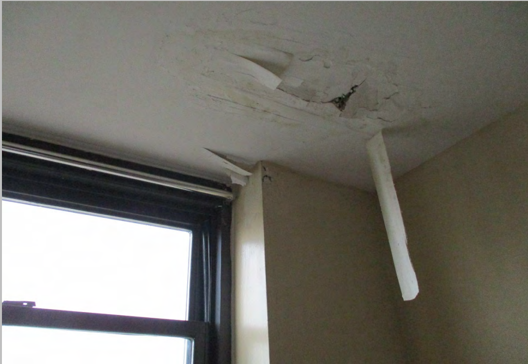
View of typical moisture intrusion in Unit 10F
