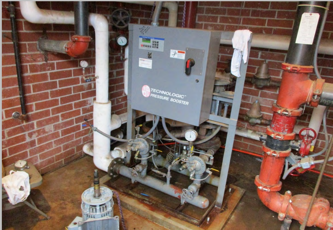
View of the pump house equipment at the subject property
