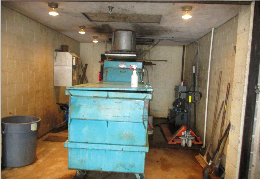
View of the hydraulic trash compactor
