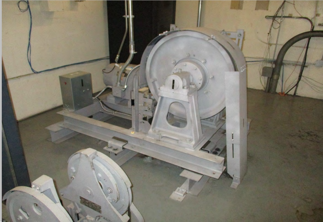
View of typical elevator equipment
