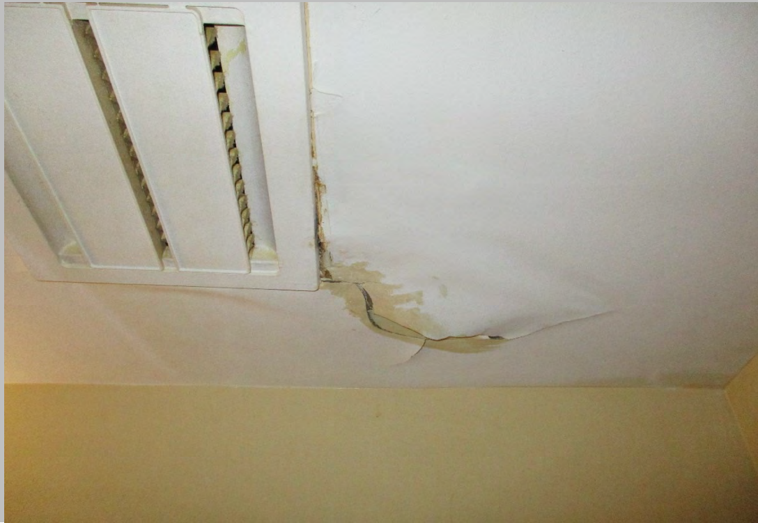
View of typical moisture intrusion in Unit 8E
