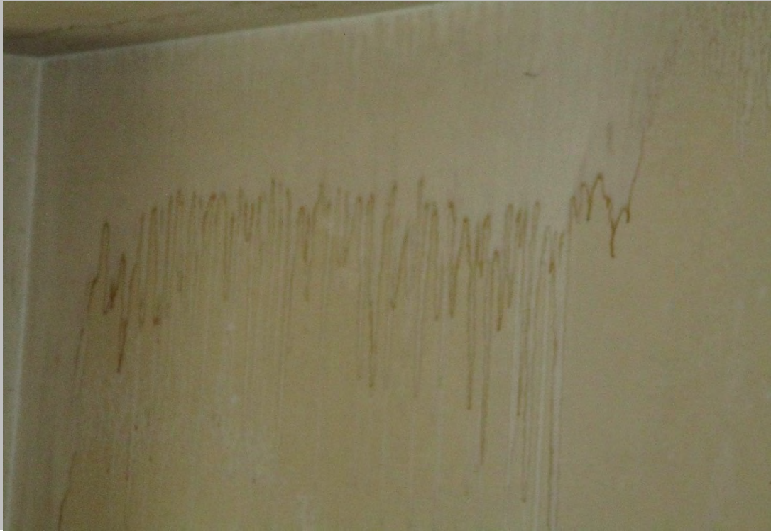
View of typical moisture intrusion in Unit 2E
