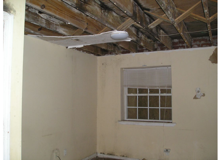
Photo 8 – Typical view of the collapsed ceiling.
