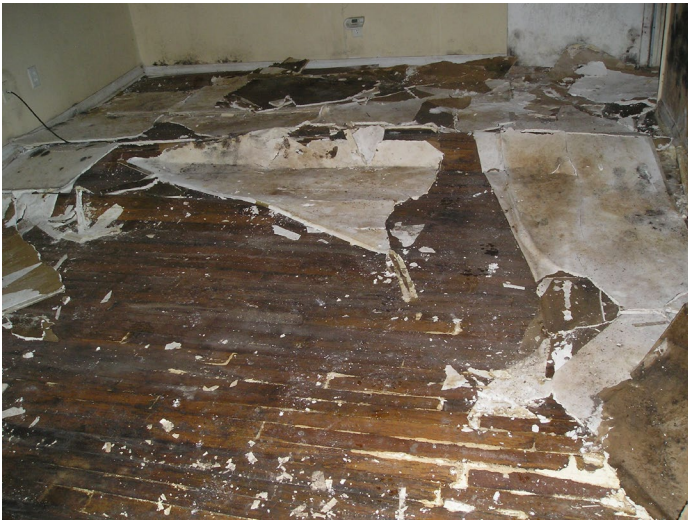
Photo 7 – Typical view of collapsed ceiling and hardwood floors.
