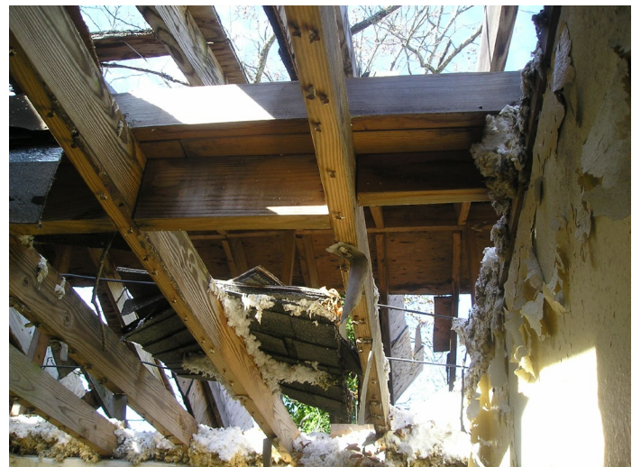
Photo 12 – Collapsed ceiling due to roof holes.
